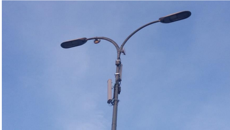
Figure 12: V2X radio equipment
